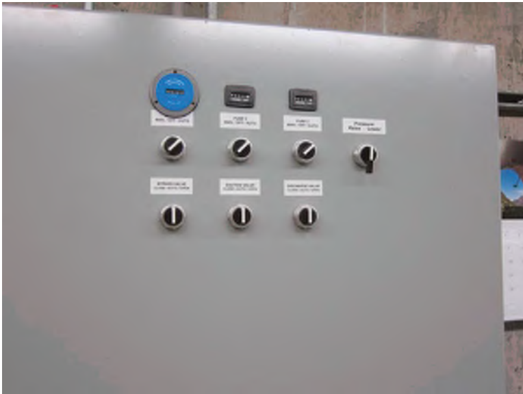
Photograph 67: Black Mountain booster pump controls
