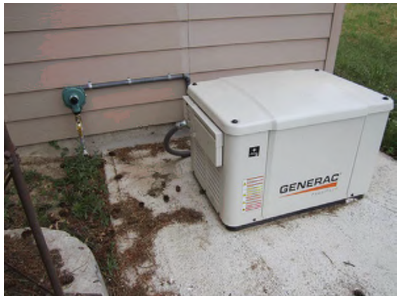
Photograph 48: Four Corners propane generator
