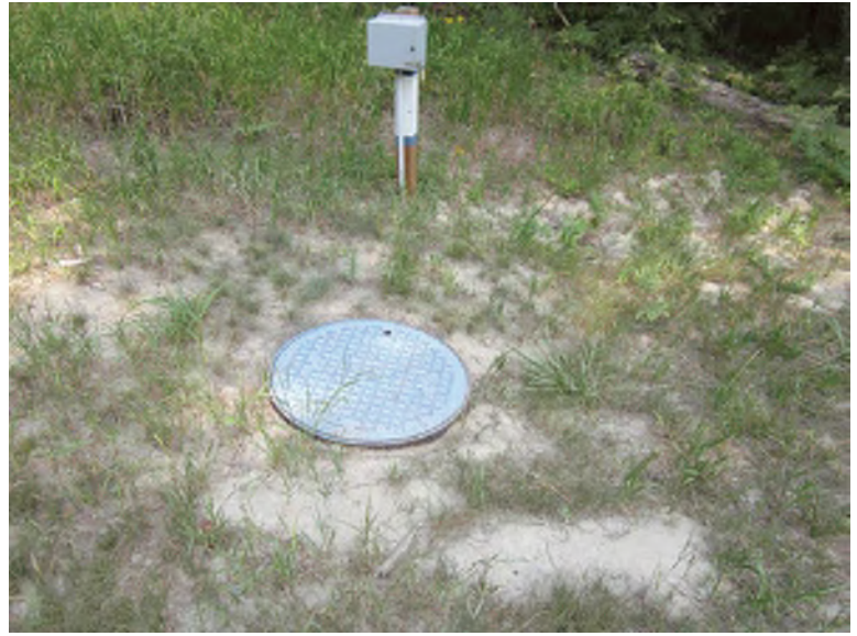
Photograph 70: Pressure reducing valve vault w pigtail
