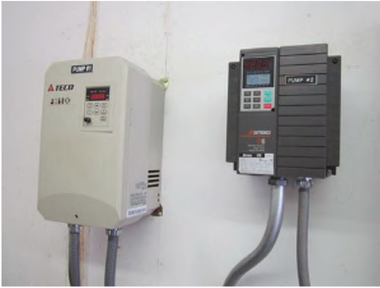
Photograph 91: Highland Flats booster pump controls
