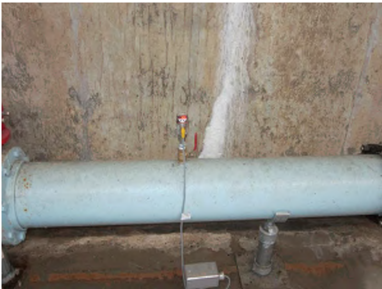
Photograph 63: Black Mountain boosted discharge appurtenances flow meter
