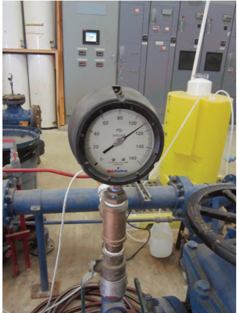
Photograph 14: Pressure gage well discharge
