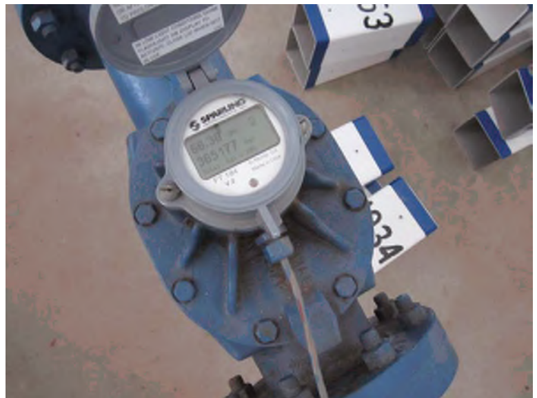
Photograph 44: Four Corners combined boosted flow meter
