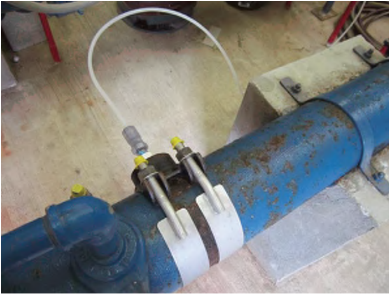
Photograph 13: Sodium hypochlorite injection quill
