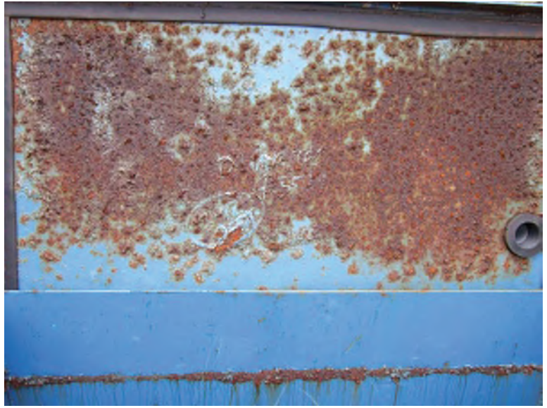
Photograph 86: Naples tank lid w water tight seal
