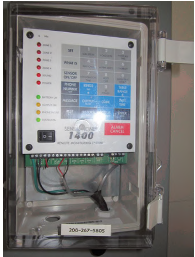
Photograph 38: Four Corners booster station autodialer
