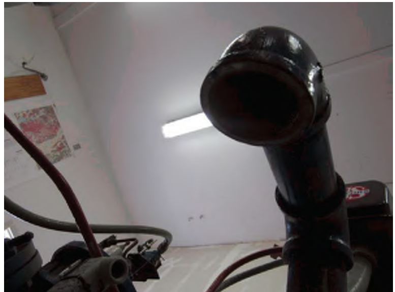
Photograph 4: Well 1 screened vent
