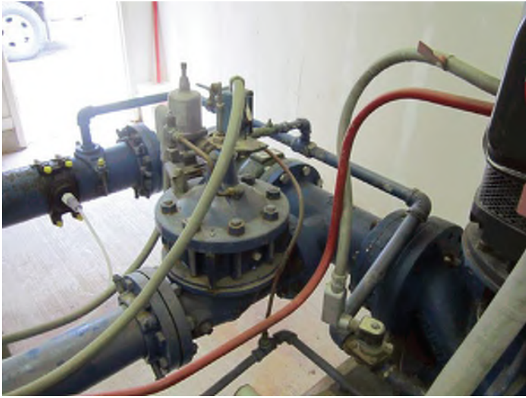
Photograph 5: Well 1 discharge to waste control valve
