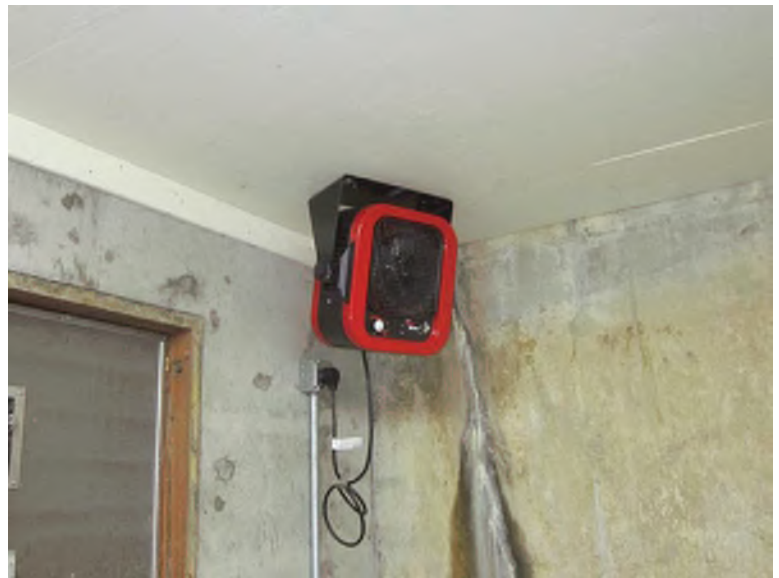
Photograph 64: Black Mountain booster station, thermostatically controlled heater
