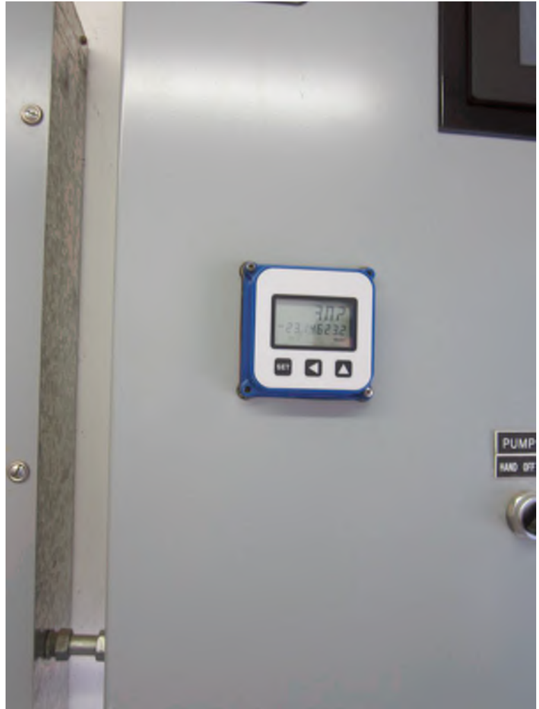
Photograph 92: Highland Flats flow meter (malfunctioning)
