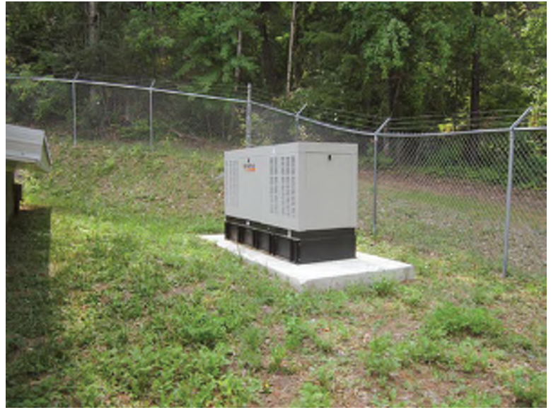
Photograph 58: Black Mountain booster station diesel generator
