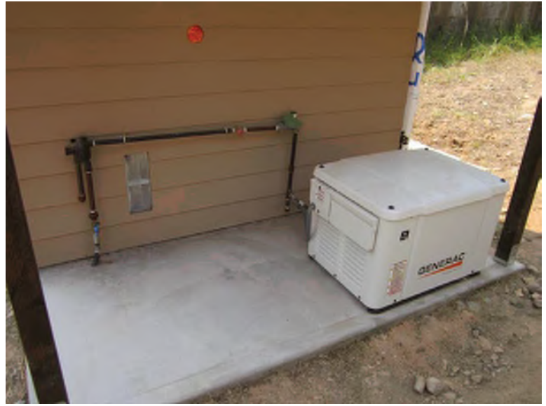
Photograph 74: Naples booster station propane generator
