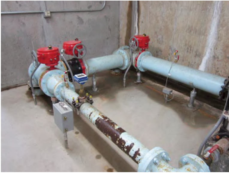
Photograph 61: Black Mountain reservoir fill line and boosted discharge appurtenances
