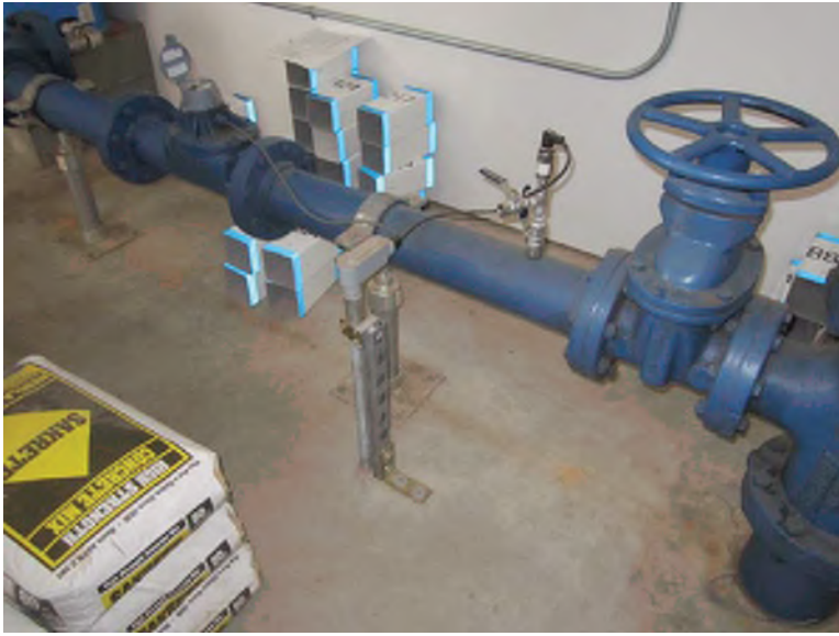
Photograph 45: Four Corners boosted discharge appurtenances
