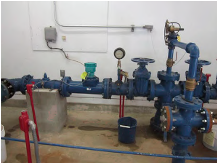
Photograph 31: Parker Canyon boosted discharge appurtenances
