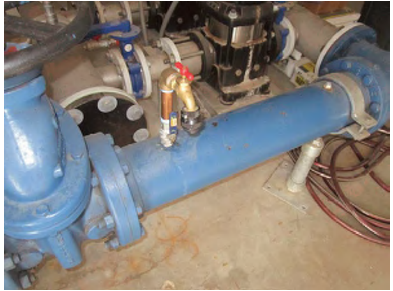
Photograph 42: Four Corners sample tap
