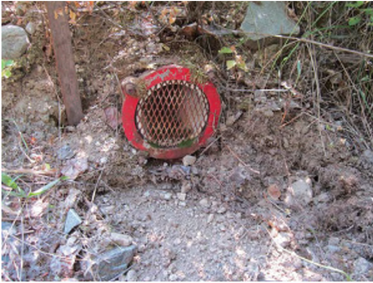
Photograph 69: Black Mountain reservoir screened overflow
