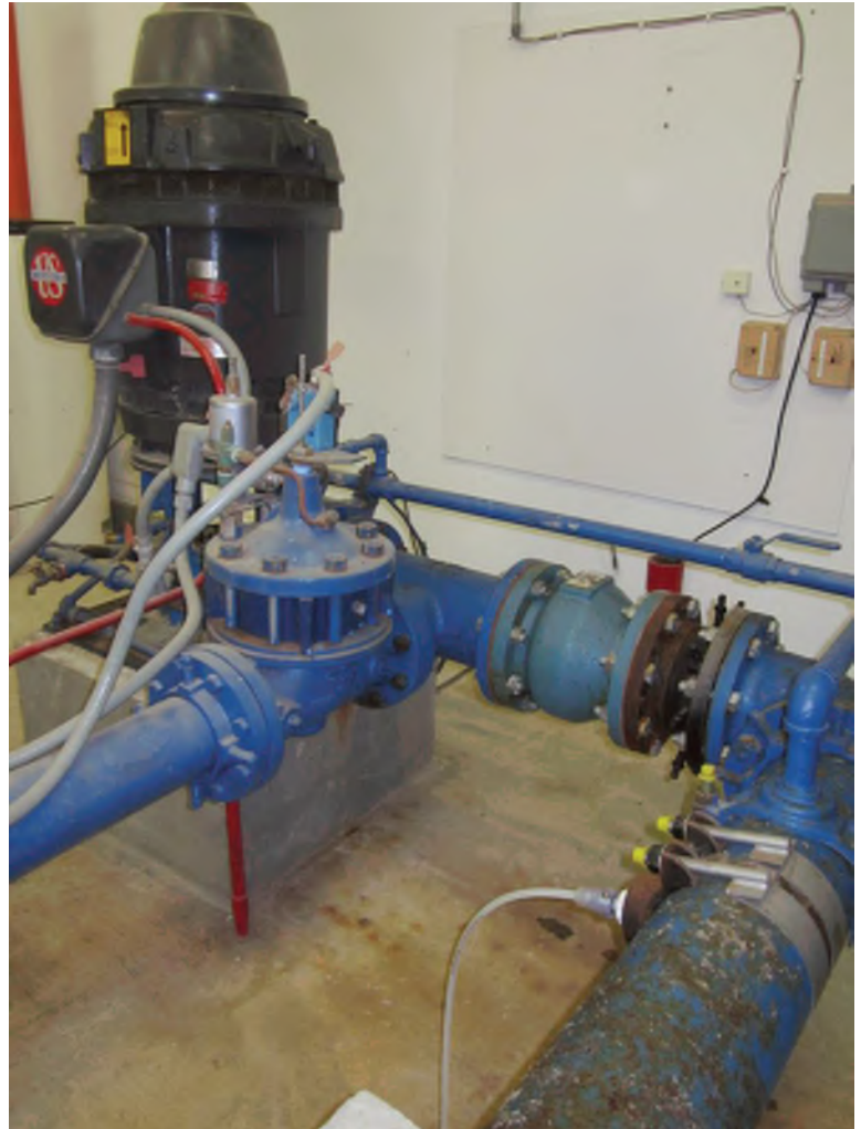
Photograph 18: Well 2 discharge to waste control valve
