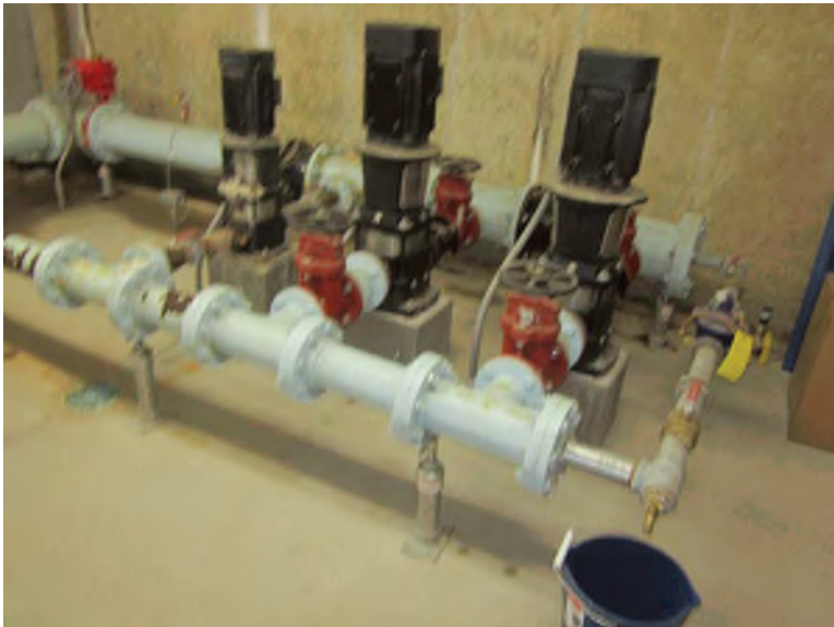
Photograph 59: Black Mountain booster pumps and discharge appurtenances
