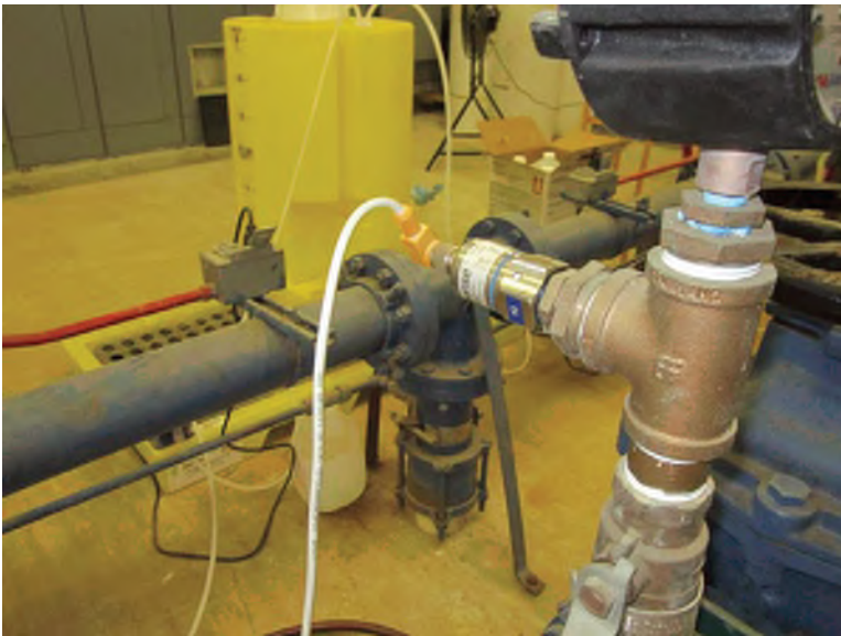
Photograph 15: Pressure transducer on combined well discharge
