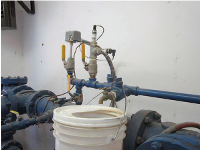
Photograph 97: Highland Flats pressure transducer and sample tap
