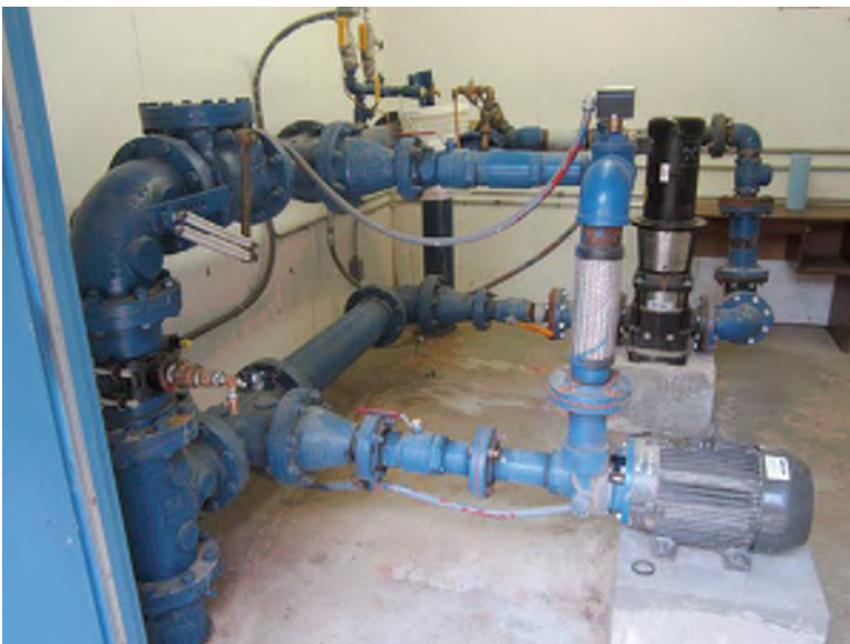
Photograph 95: Highland Flats boosted discharge appurtenances
