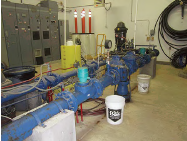
Photograph 1: Well discharge appurtenances
