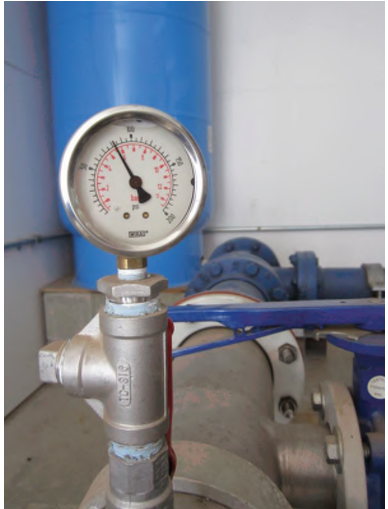
Photograph 46: Four Corners inlet pressure
