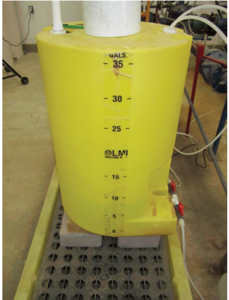
Photograph 10: Sodium hypochlorite day tank
