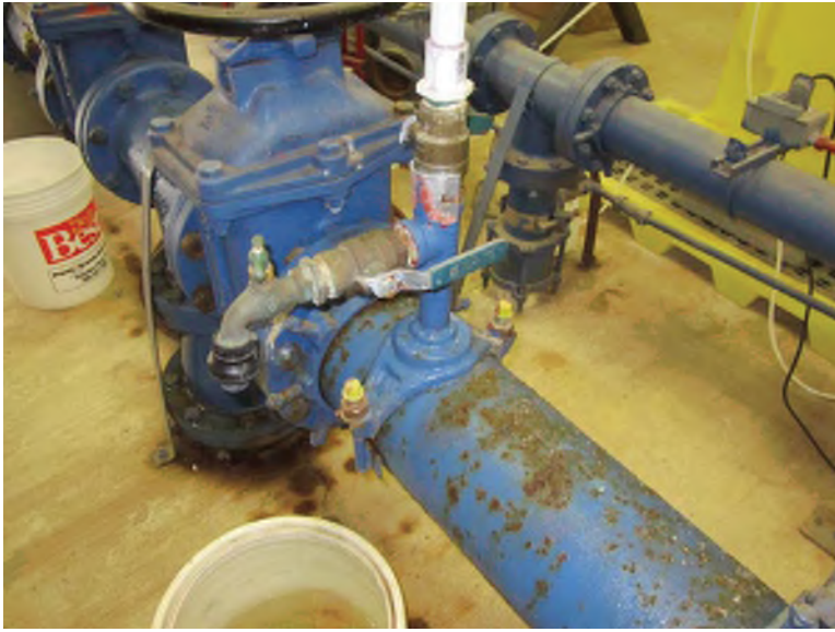
Photograph 17: Finished (chlorinated) sample tap
