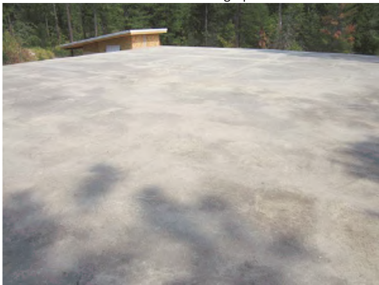
Photograph 81: Naples tank roof
