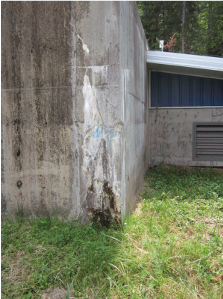
Photograph 49: Black Mountain reservoir (leak)
