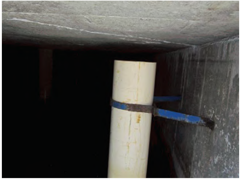
Photograph 54: Black Mountain reservoir interior overflow
