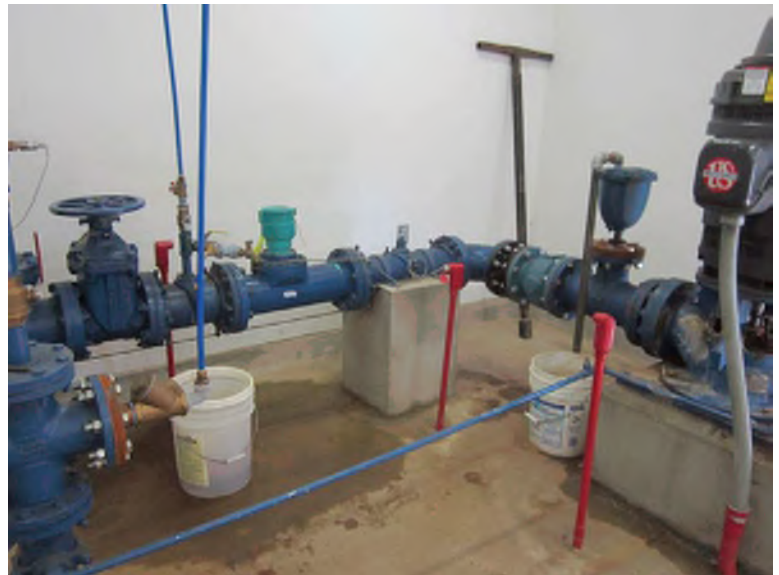
Photograph 32: Parker Canyon boosted discharge appurtenances
