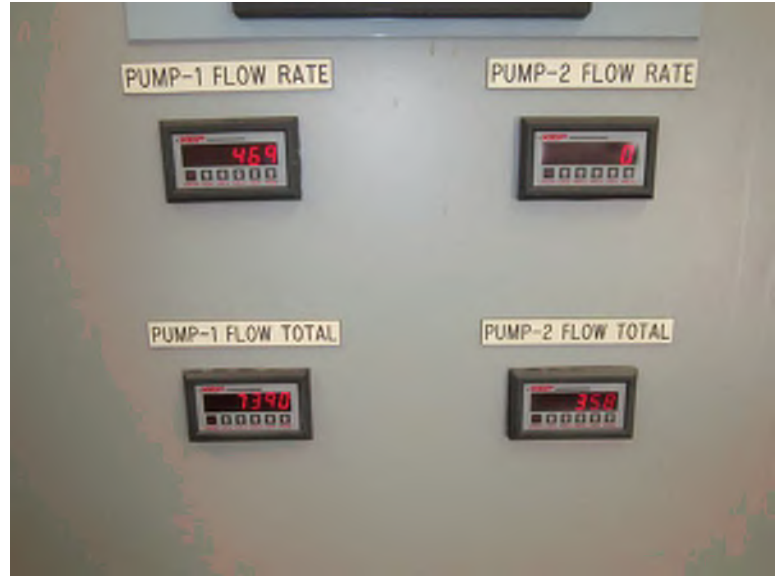
Photograph 34: Parker Canyon pump controls
