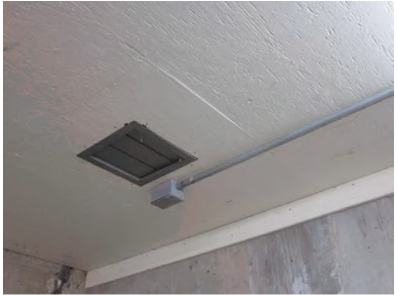
Photograph 66: Black Mountain booster station, thermostatically controlled louvre vent
