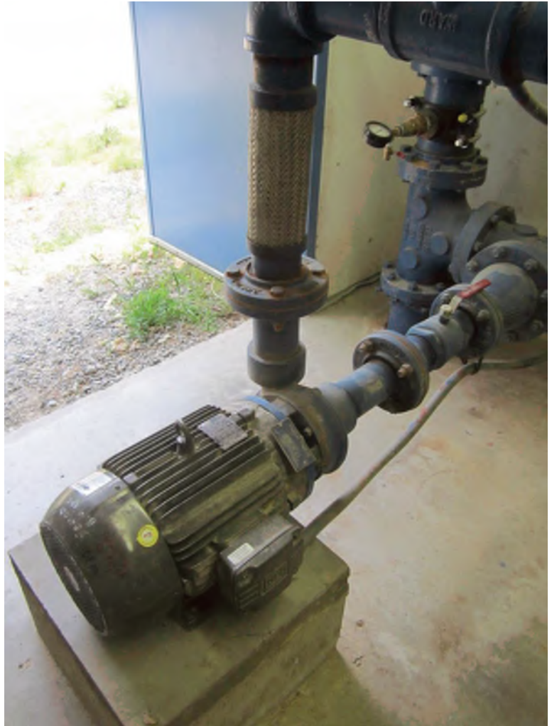
Photograph 98: Highland Flats booster pump
