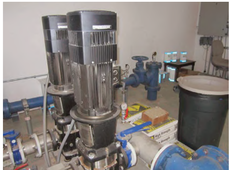
Photograph 40: Four Corners booster pumps and discharge appurtenances
