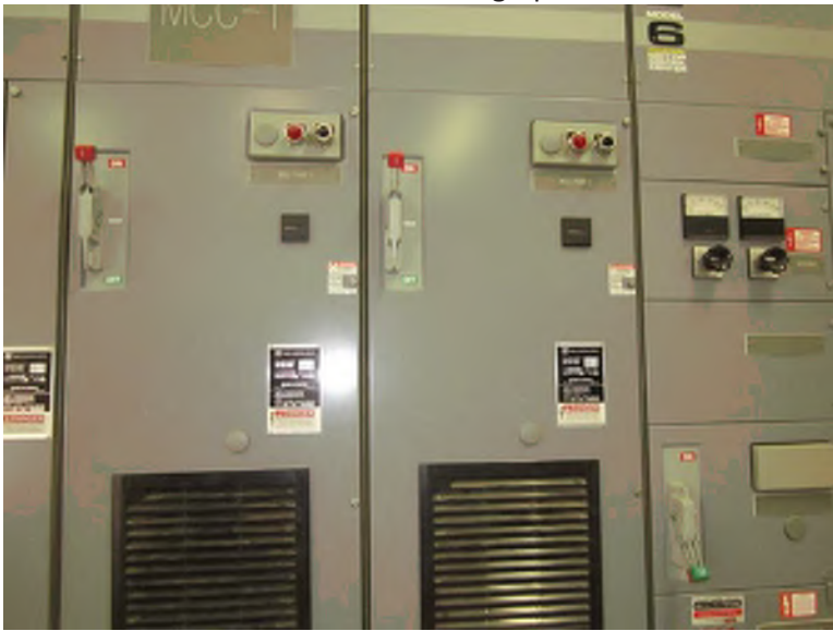
Photograph 19: Well electrical switches
