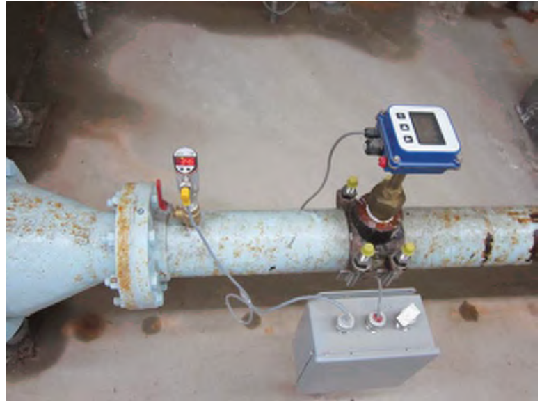
Photograph 62: Black Mountain boosted discharge flow meter
