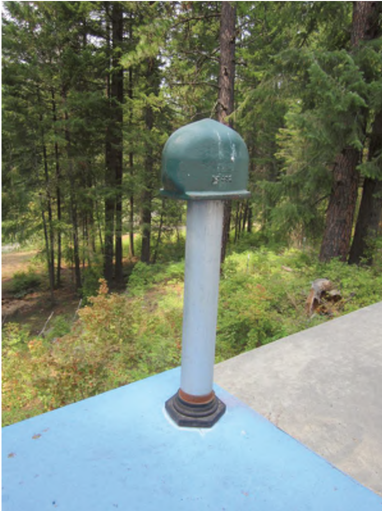
Photograph 87: Naples tank lid w screened vent
