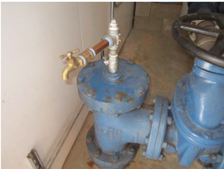
Photograph 43: Four Corners sample tap
