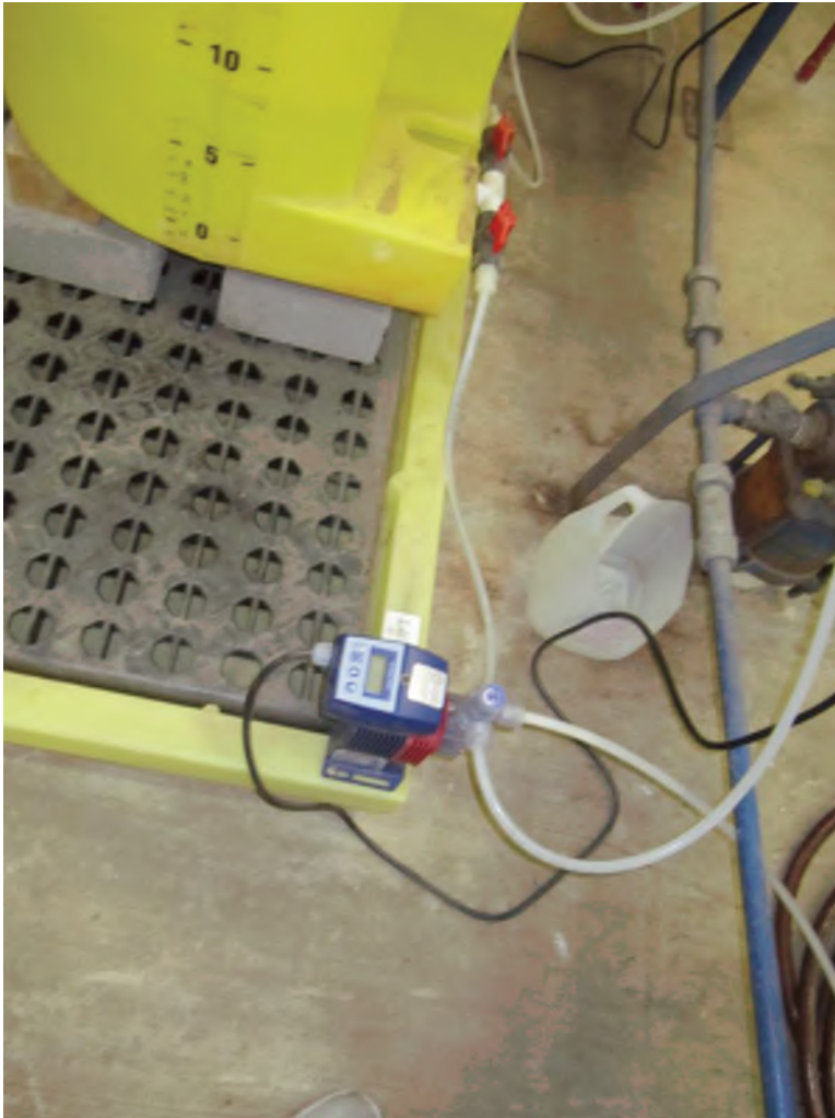
Photograph 11: Well 1 electronic metering pump
