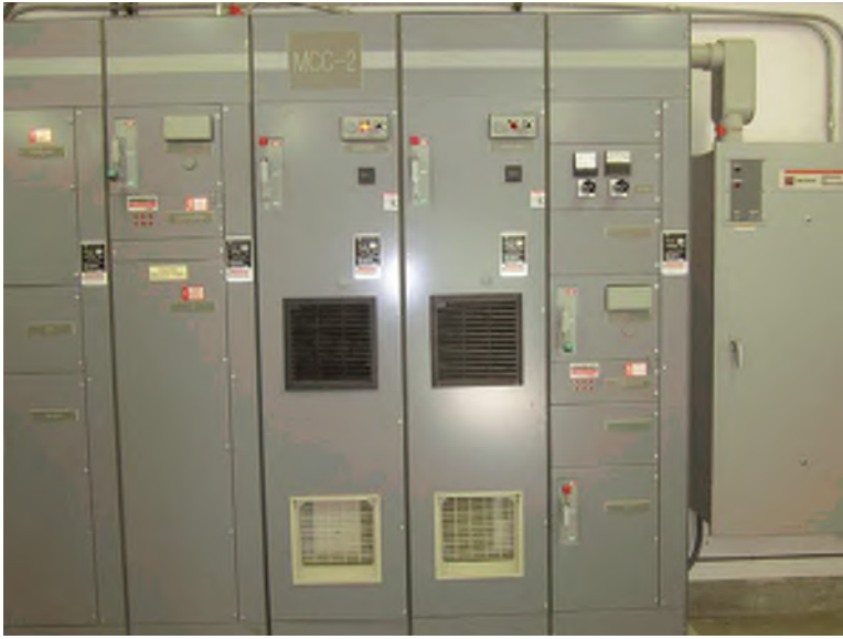
Photograph 33: Parker Canyon booster pump controls
