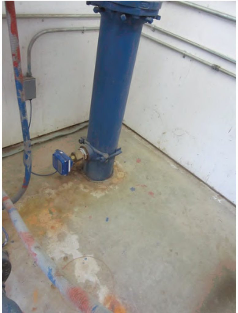
Photograph 94: Highland Flats combined boosted discharge flow meter
