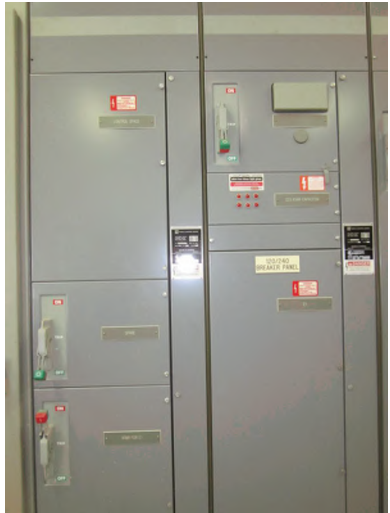
Photograph 20: Well electrical switches
