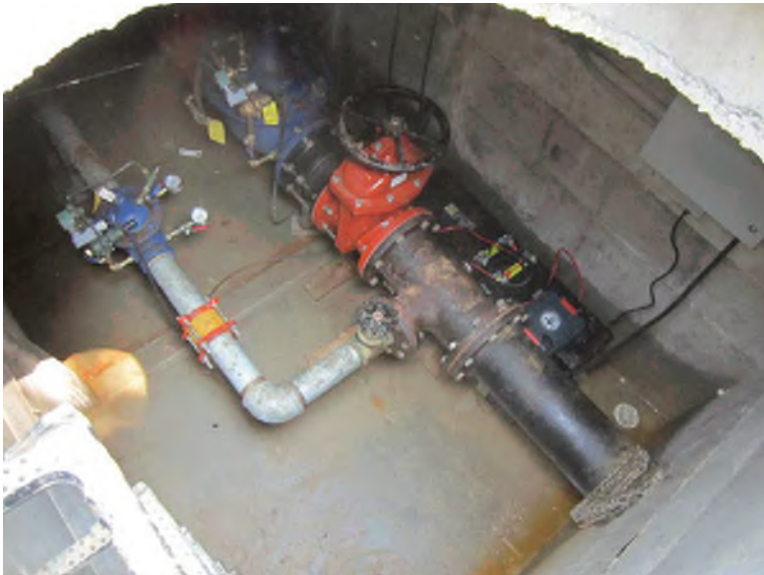
Photograph 71: Pressure reducing valve vault
