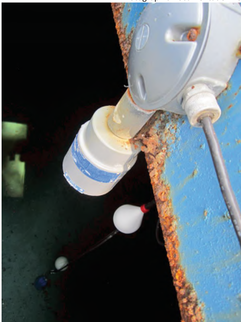
Photograph 83: Naples tank ultra-sonic level transducer
