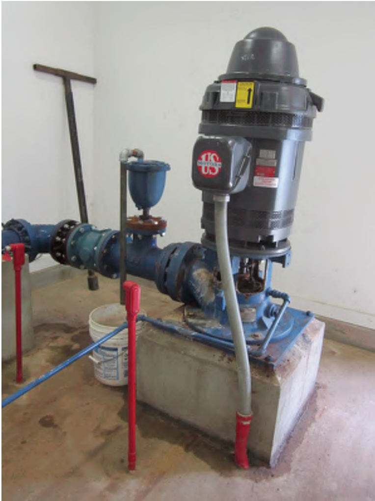
Photograph 29: Parker Canyon booster pump
