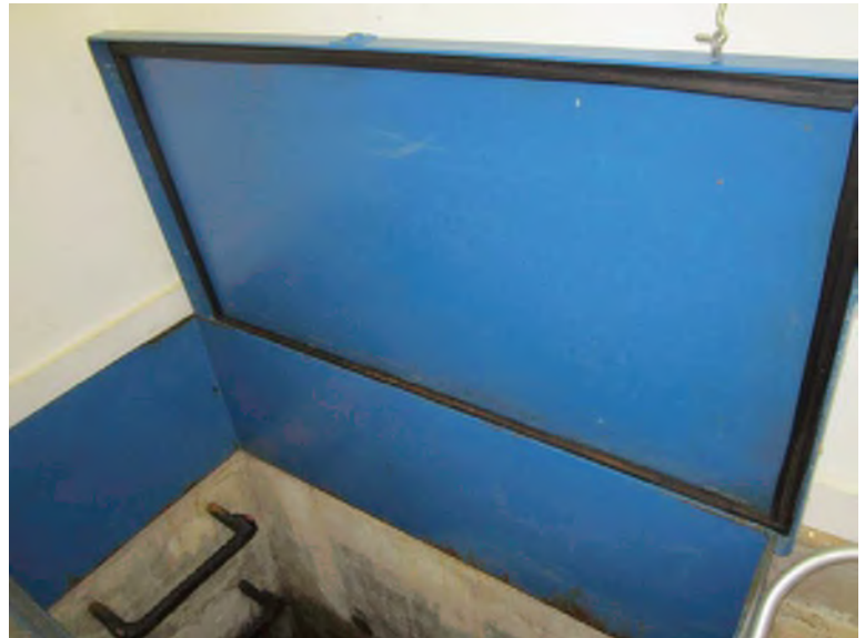
Photograph 28: Parker Canyon tank water tight access hatch
