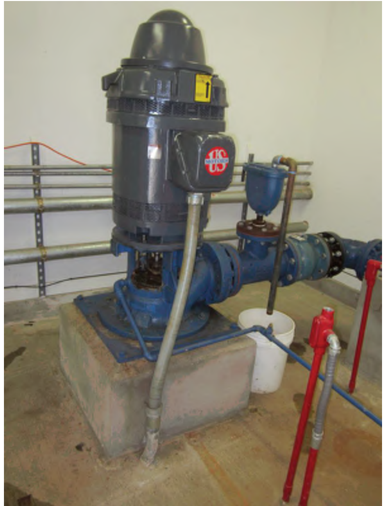
Photograph 30: Parker Canyon booster pump
