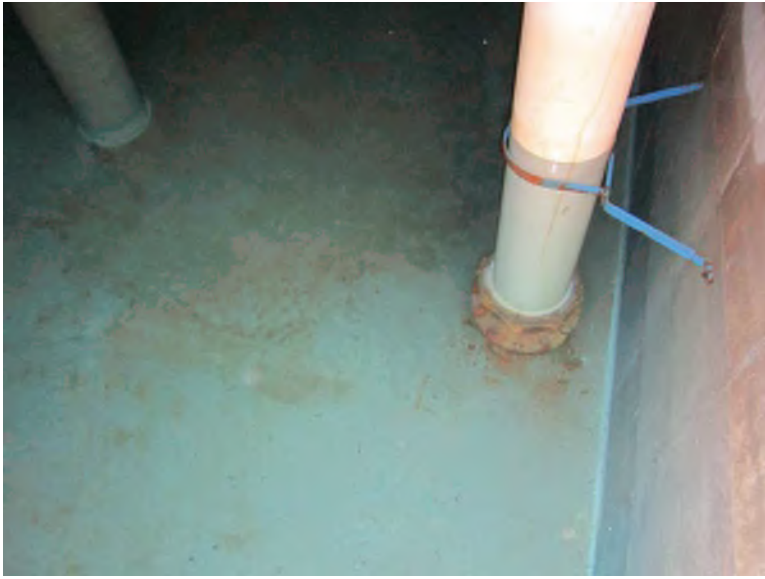
Photograph 53: Black Mountain reservoir interior overflow
