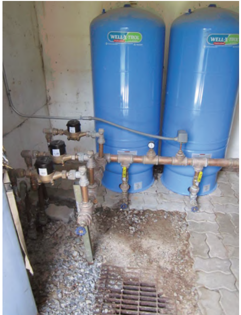
Photograph 76: Naples tank booster station, 3 residential connections
