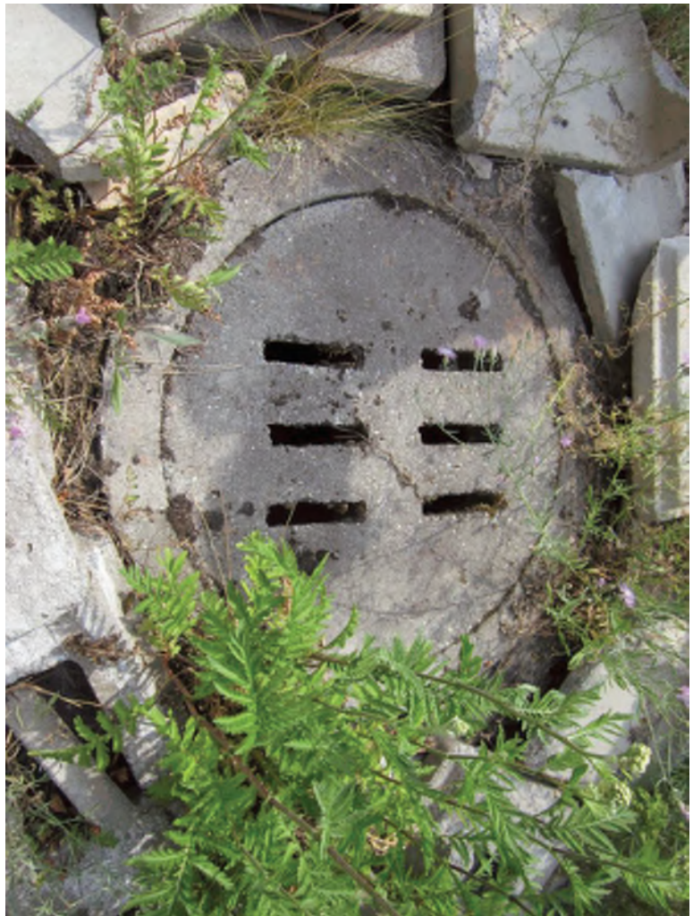
Photograph 22: Well discharge to waste dry well (requires air gap/backflow protection)
