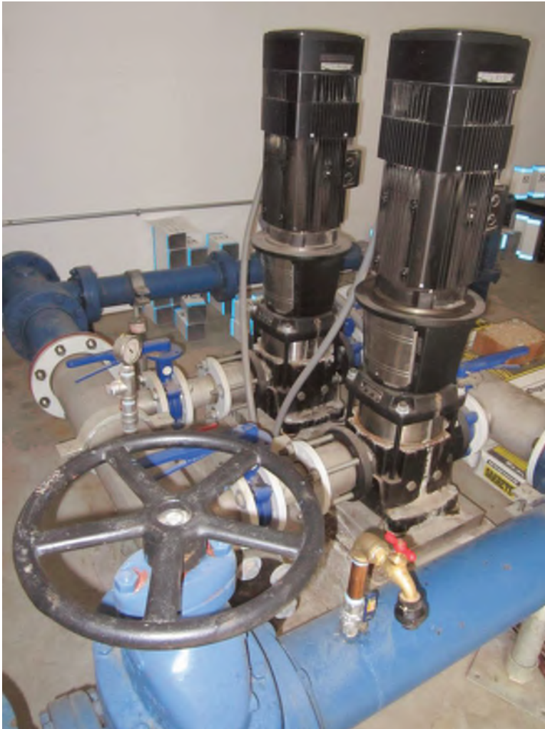
Photograph 41: Four Corners booster pumps and discharge appurtenances
