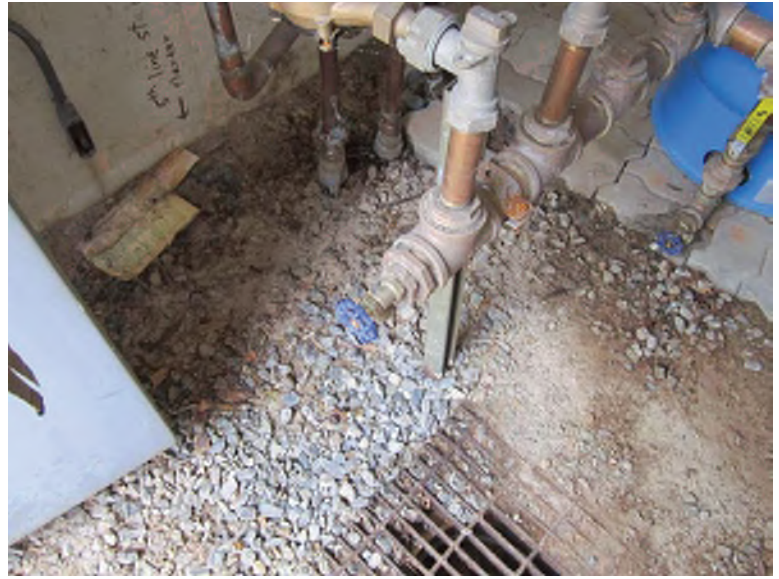
Photograph 78: Metered residential connection w corp stop
