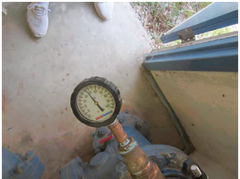
Photograph 96: Highland Flats inlet pressure
