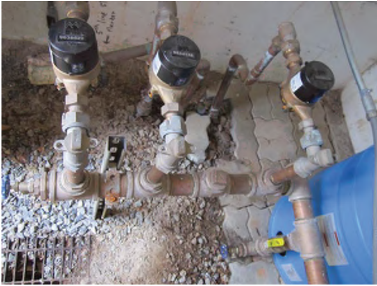
Photograph 77: Naples tank boosted discharge, 3 residential connections
