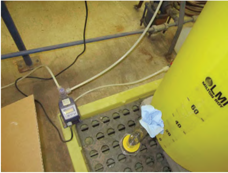
Photograph 9: Well 2 electronic metering pump and calibration cylinder
