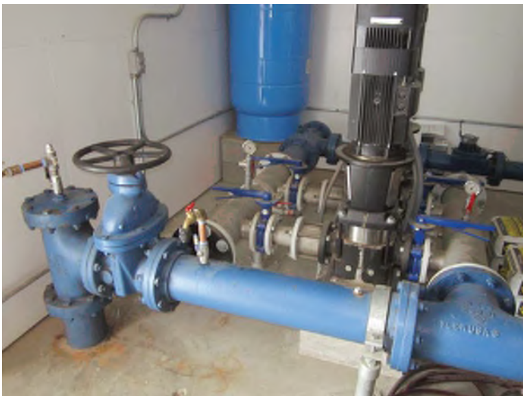
Photograph 39: Four Corners booster station
