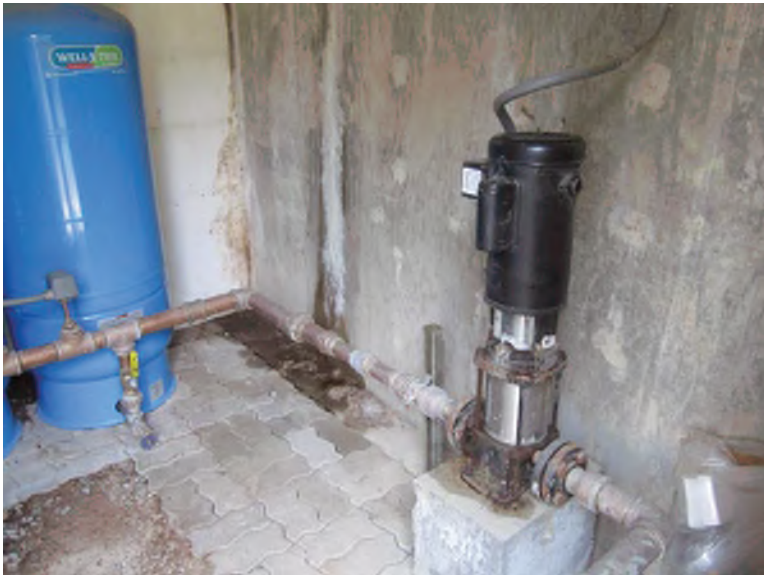
Photograph 75: Naples tank booster pump
