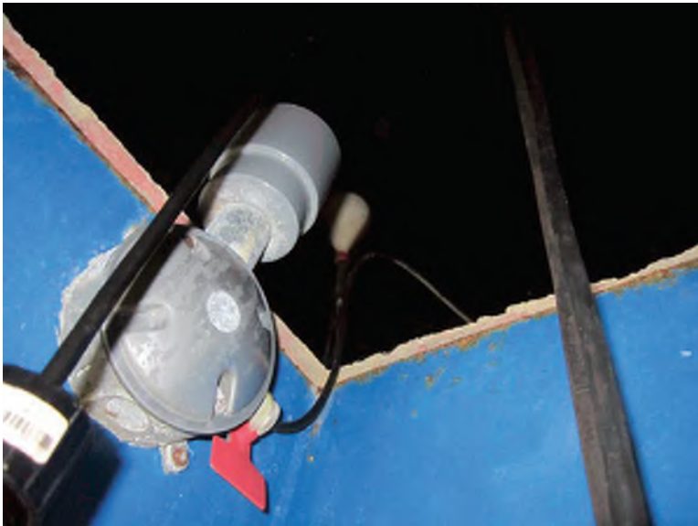
Photograph 27: Parker Canyon level controls (well actuation)
